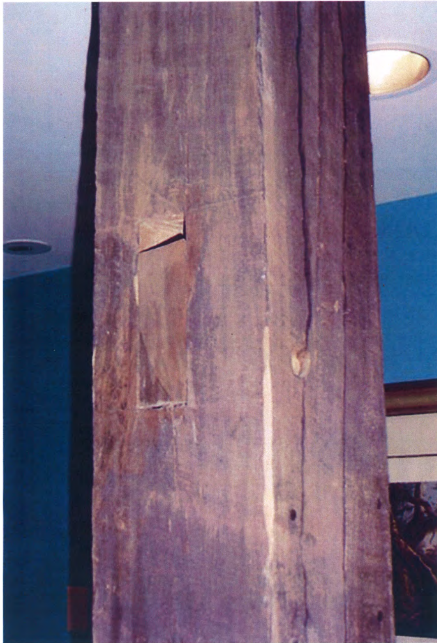
Figure 3. Detail of mortise, tenon, and peg in heavy-timber post on third floor. WLS, 2004.
