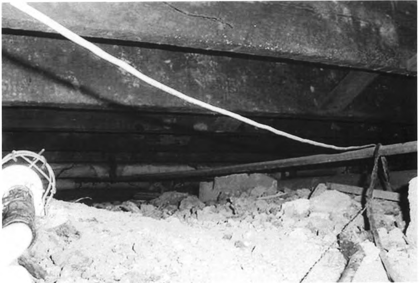
Figure 25. Floor joists under center stair hall. Note vertical saw marks on the second joist. WLS, 2004.
