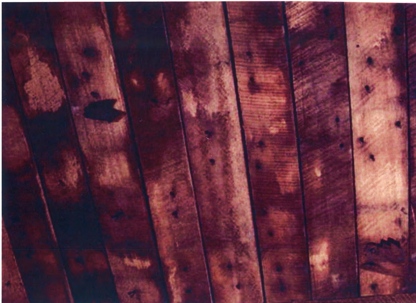
Figure 74. Reused sheathing boards with nail and fragments of wood shingles on the undersides. Located in the south garret on the 3 rd floor. WLS, 2004.
