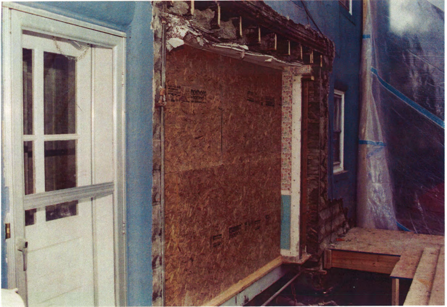
Figure 35. South façade after removal of original maid's room bay. Note the heavy-timber barn beam above the opening and the concrete block walls behind the stucco finish. T. Mueller. 1993.
